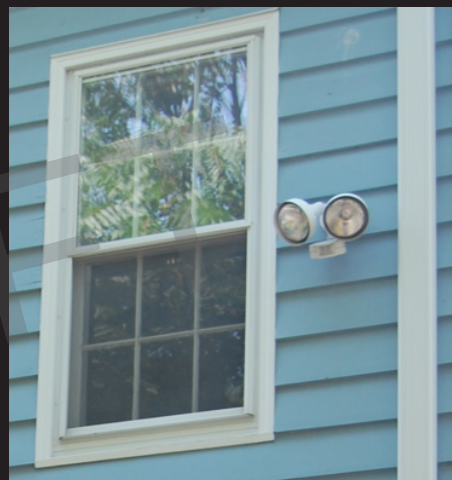
This is an example of a minimally visible security light fixture.
