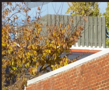
Example of appropriate roof-mounted HVAC screening.
