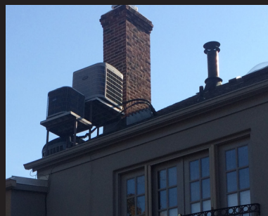
Example of inappropriate unscreened roof-mounted HVAC.
