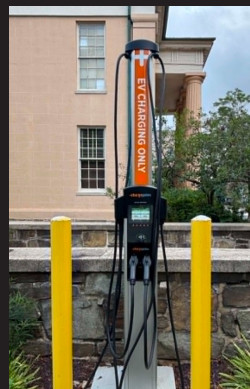
Example of an electric vehicle charging station.
