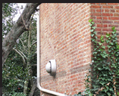
Example of inappropriate piping installed on a visible facade.
